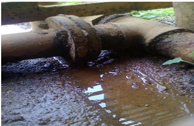
Plate 1: Leakage from the burst pipeline
